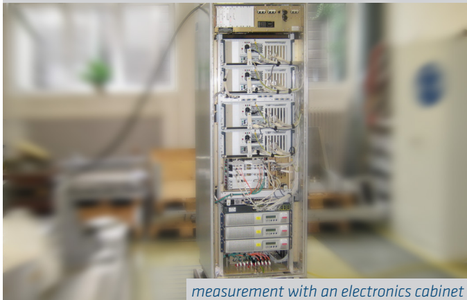
measurement with an electronics cabinet
